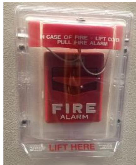
FIRE ALARM PULL STATION
