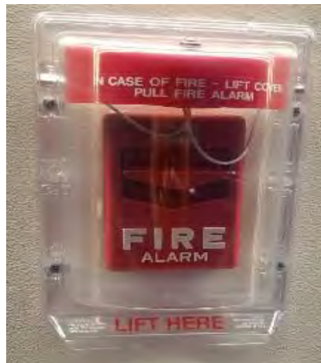
FIRE ALARM PULL STATION
